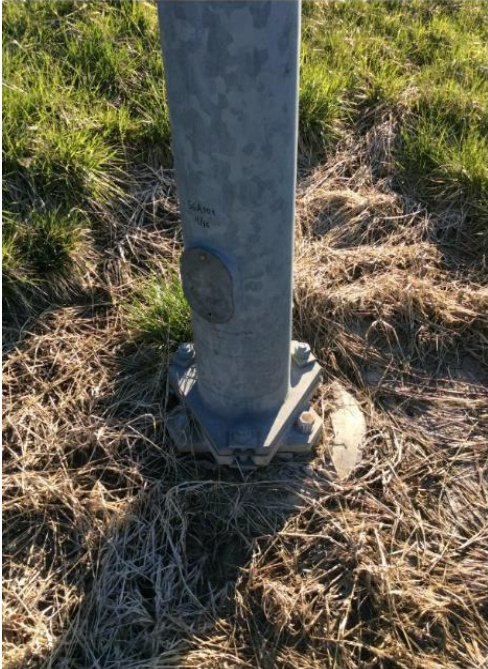
Door in place, electronics in good condition
