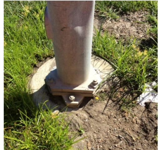
Poor – deteriorated, damaged, consider for repair – fix in project
