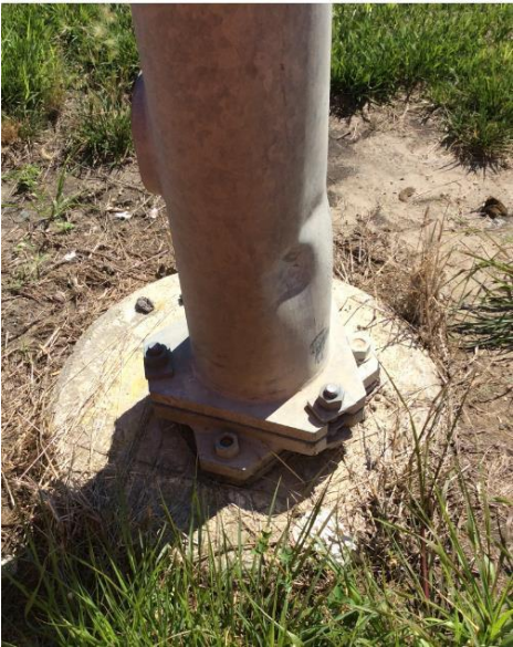
Damage to pole
