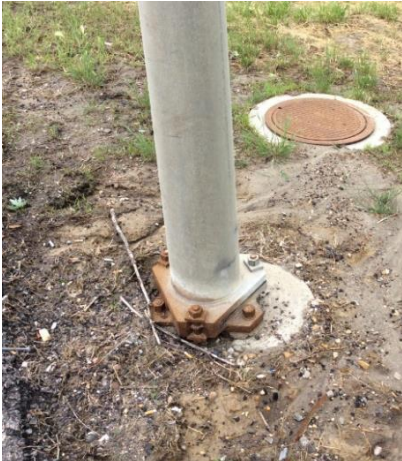
Rust on pole or mast arm.
