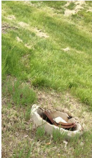
Very Poor – Serious Deterioration/Damage – fix as soon as possible
