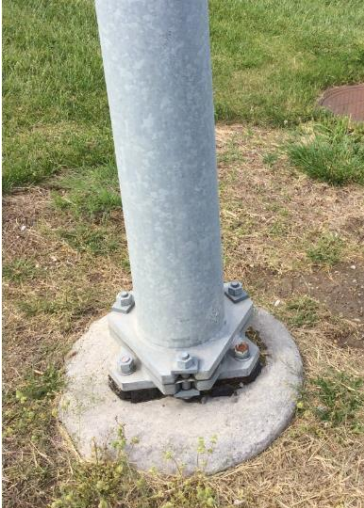
No rust/Damage, all bolts in place
