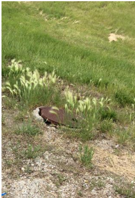
Poor - Deteriorated/Damaged, consider for repair or replacement
