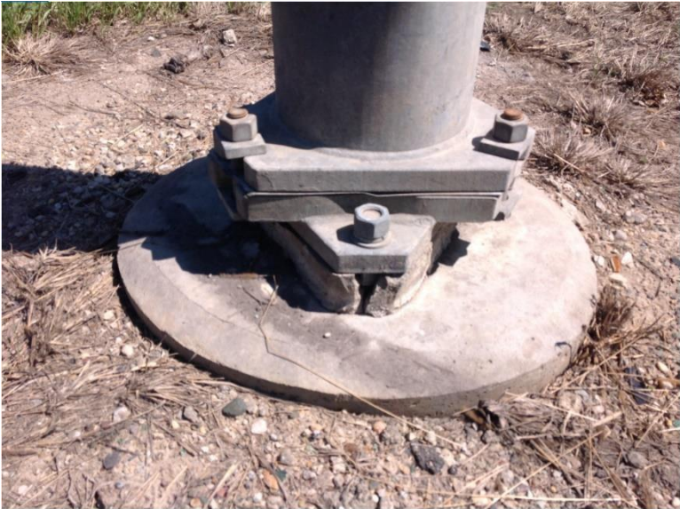
Slip plate torked, loose or missing (where applicable)
